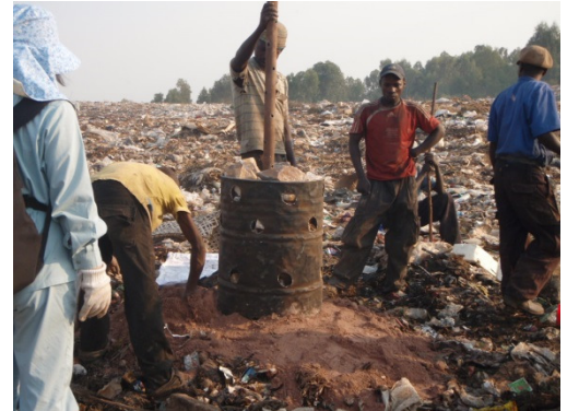
Installation of a gas ventilation system at Nyanza landfill based on the Fukuoka Method with an expert group from Fukuoka University in Japan (July 2009)
