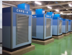
After the training, I also visited a facility to generate electricity from collected organic waste ('Recyclean' in Takigawa city, Hokkaido)
