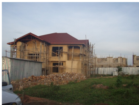
Huge house under construction in Kigali キガリ市内の建設途中の邸宅
