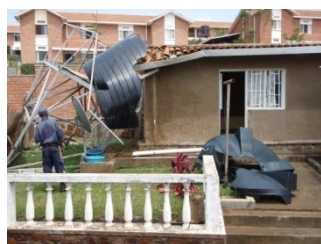
Dec – Collapsed water tank
